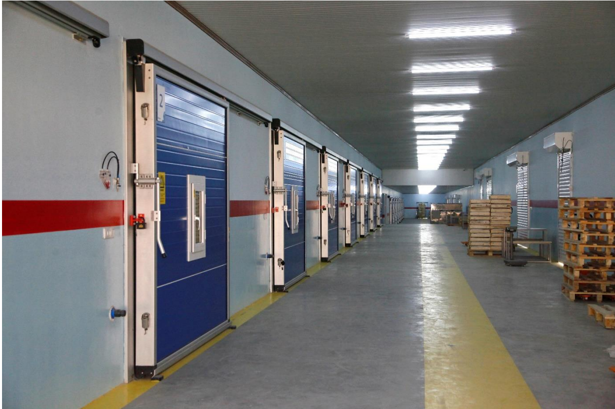
Cold stores from a Geerlofs project
